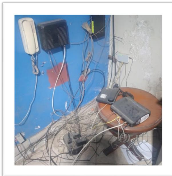
Figura 32: Switch y Router
